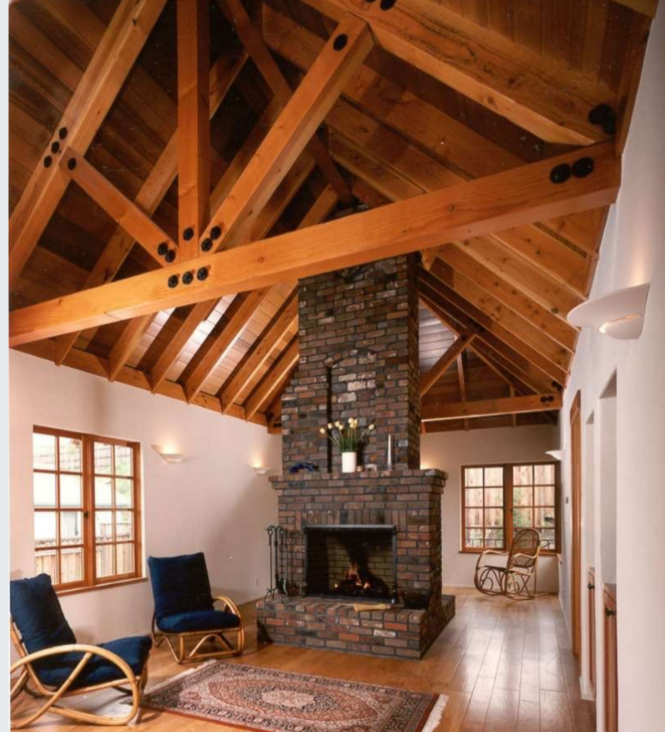
A rebuilt and better version of the chimney rises through the middle of the living room with no adjacent walls. Photo: Allen Geller
